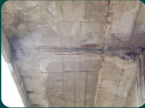
Šibenik Bridge: deterioration at the underside of bridge deck
