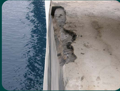
Pag: delamination at the edge of the arch abutment
