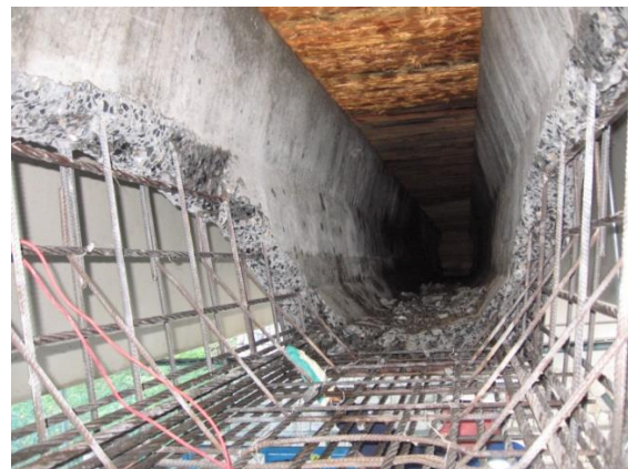
Figure 2: Damage within the beam following hydrodemolition.
